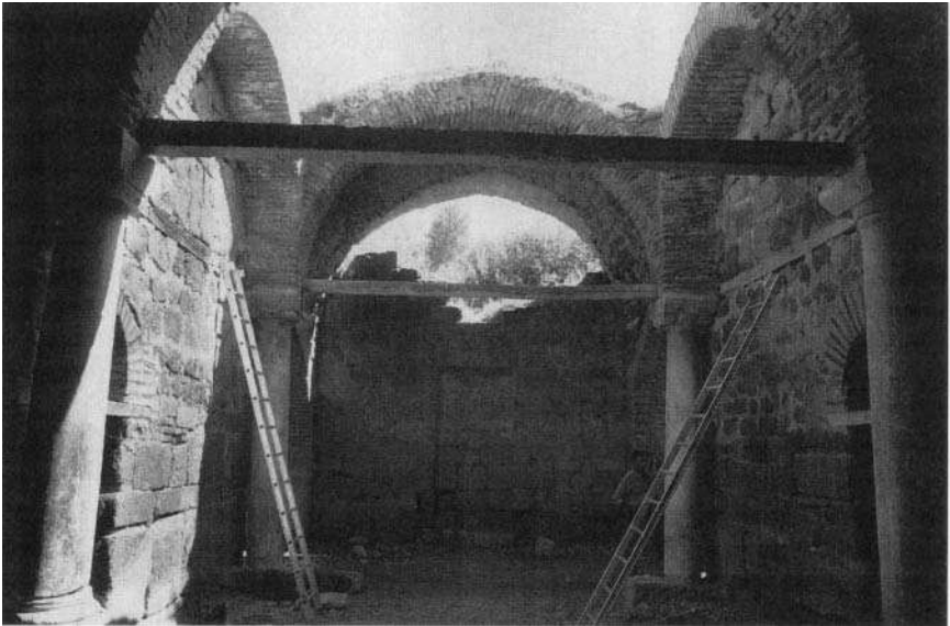
Figure 4.20. Afyon, Sincanlı, Boyaliköy Medresesi, interior. The oak tie-beams, wall-stretchers, and door-lintels were cut in 1206. The “beam” in the foreground is a poured concrete replacement. (P. I. Kuniholm, ADP)
